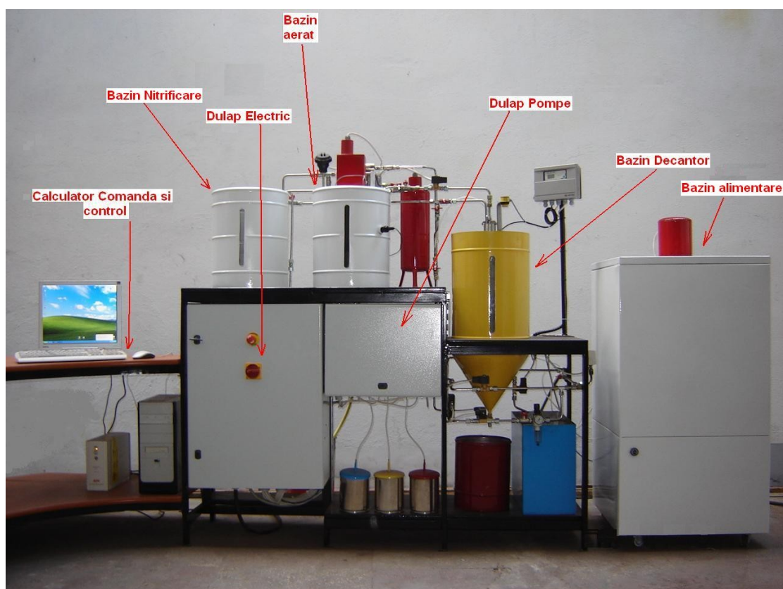
Figura 2: Statia pilot de epurare biologica
